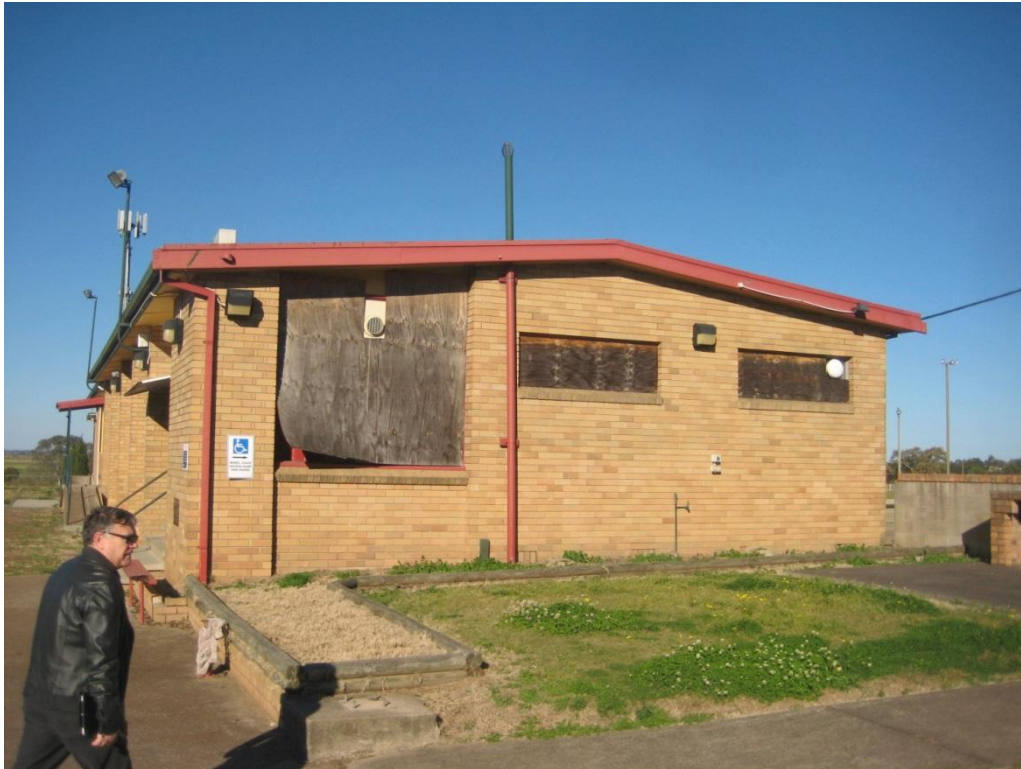
Figure 14. The former clubhouse from the west. Note signs of illegal entry. EJE
